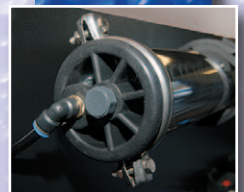
RO membrane stainless steel housing
